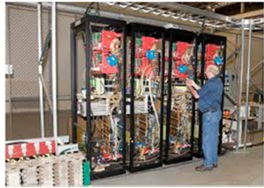
Fig. 23. Solid-state transformer based on 15 kV SiC MOSFET [95].
