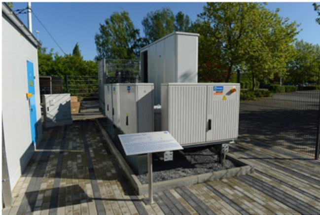
Fig. 16. GE 1MW SiC inverter installed in Berlin.
